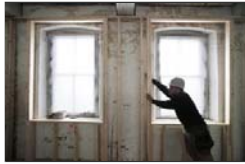
Larry Mitchell puts up a stud wall in The Mill at Saco Falls. Forty of the 66 units being built will be reserved for people earning 50 percent or less of the area's median income.
