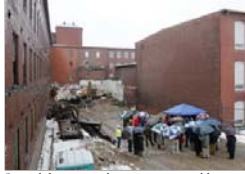
Several dozen people turn out at an old Biddeford mill Monday for the groundbreaking of a Maine Workforce Housing conversion project. The mill being converted is in the background on the right.
